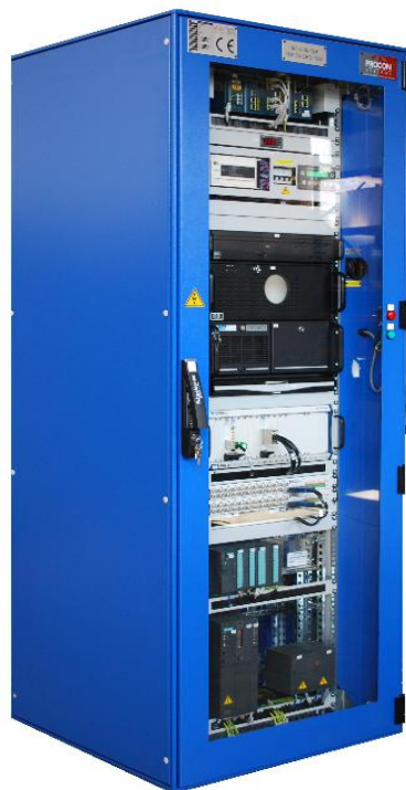
Figure 1: Illustration of a Magnet control cubicle
